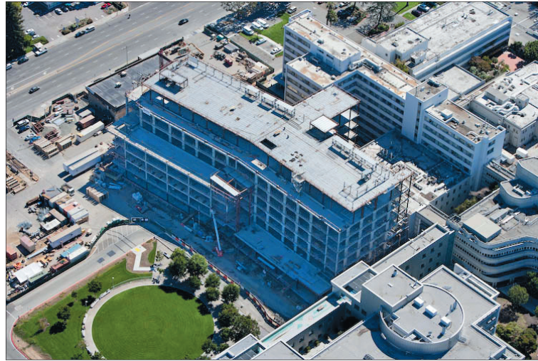
Construction on the Sobrato Pavilion started just a few months after the passage of Measure A in November 2008, a significant feat given the complexity of the building.
